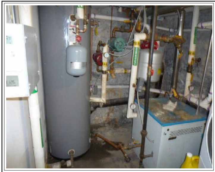
Boiler and Hot water heater
