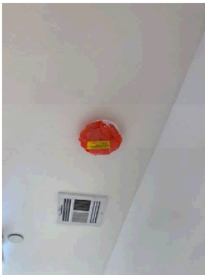
SUBJECT UNIT CO/SMOKE DETECTOR
